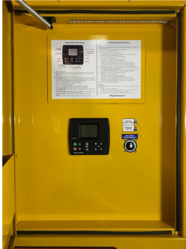
Figure 1: ES-FLS control panel
